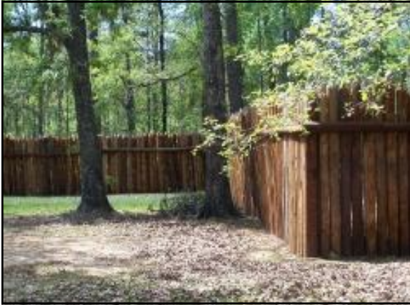
Part of the Restoration Projects Ongoing at Fort Mims, this is a section of the restored stockade walls.
